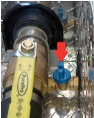
Shut off valve for foam
